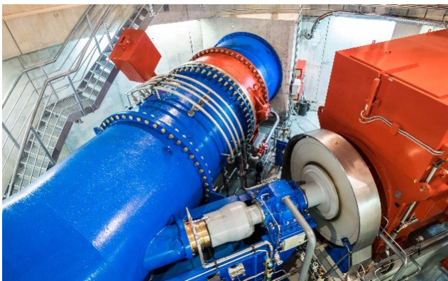
Hydropower application example
