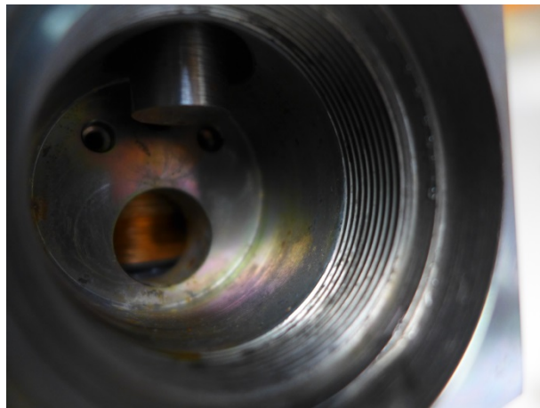
Result: No water was found in the unit under test number 4
